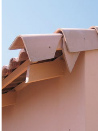
GOODBYE MR CHIPS: Occupiers could find themselves saying hello to the repair bill for this damaged roof tile if they fail to read the contract's small print
