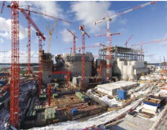
This European Pressurised Water Reactor under construction in Olkiluoto, Finland, by Areva-Siemens France, is similar to the ones under discussion for Bantamsklip
