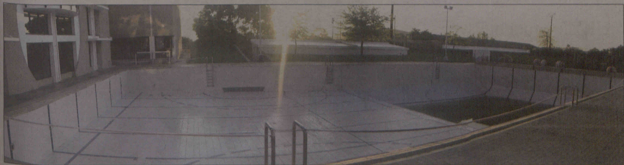
SWIMMING UPSTREAM Stellenbosch University's outdoor swimming pool has been empty since May 2010 in order to repair a leak. Apparently, no repairs have been made as of yet. The pool is the practice pool for the SU water polo and underwater hockey teams. Photo: LIDA-MARI GROENEWALD
