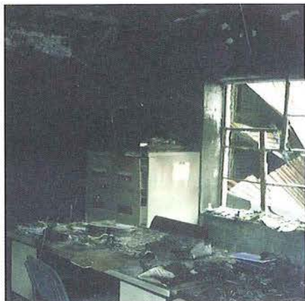
Fire damage at MBV Spares
