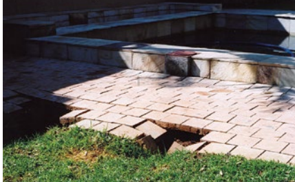
Fallback position: Collapsing brickwork alongside the pool
