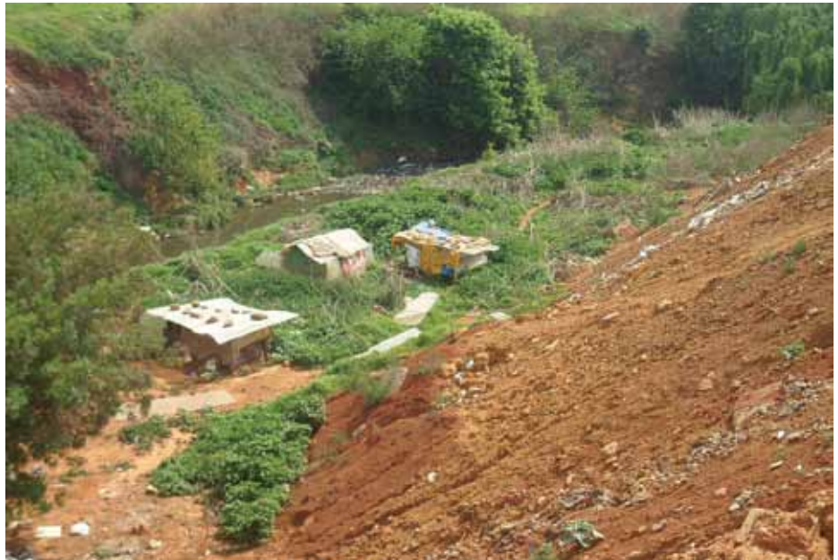
Living dangerously The dump from excavations at the Oriental City site pose a serious threat to shack dwellers, who risk a landslide from the mountain of earth
